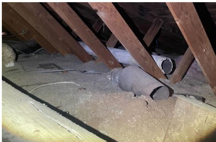
Example of the condition of a home attic before EASE Home upgrade includes fully disconnected ducts with asbestos and signs of rodent activity.
