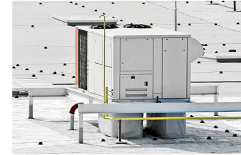
Efficient Rooftop Units
